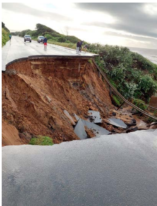
Above: Scenes from the flooding in KwaZulu-Natal. Opposite page: Learners from The Green School survey the debris the waters left after washing away a large section of the road surface.
